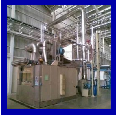
SS Ducting Systems
