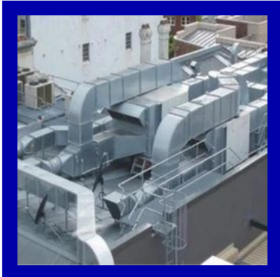
Exhaust Ducting System
