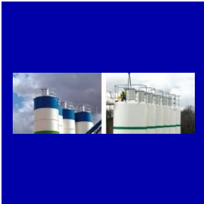
Silo Venting Filter
