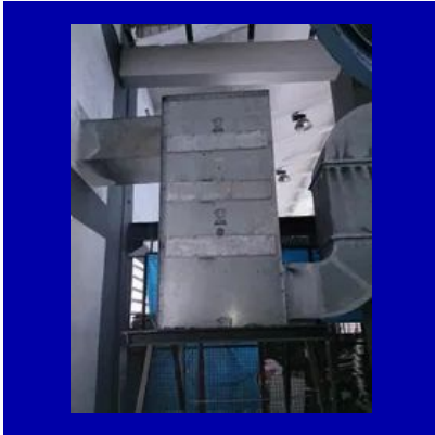
Paint Booth Scrubber
