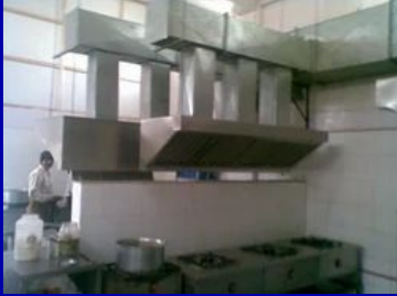
Kitchen Exhaust System
