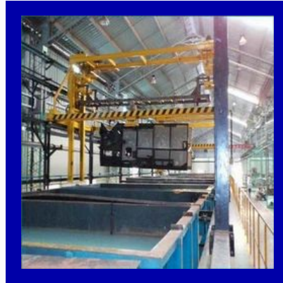
Dip Pretreatment Plant
