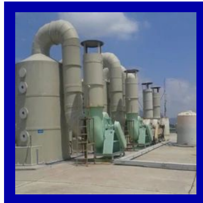
Activated Carbon Tower
