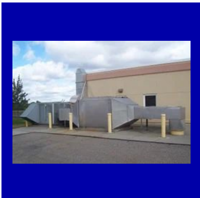
Odour Control Scrubber
