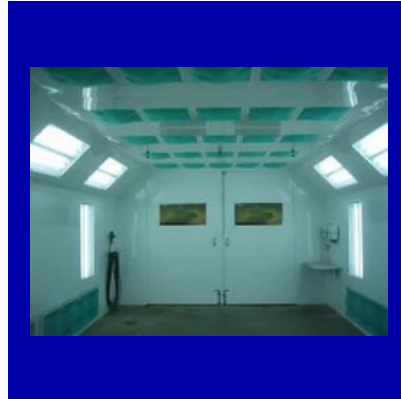
Paint Booth Roof Filter
