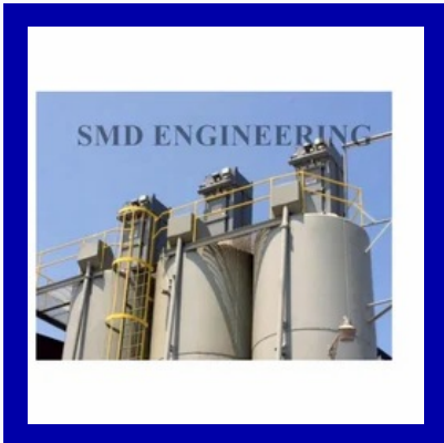
Bin Vent Filter
